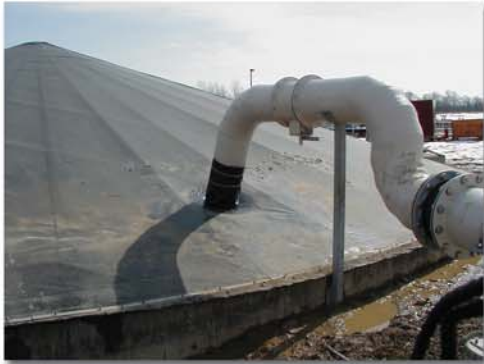
ODOR CONTROL DUCTWORK
